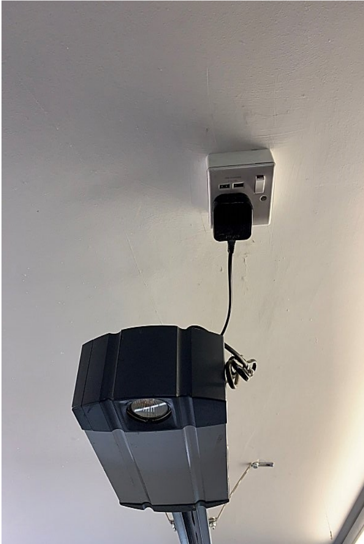
Pic C shows unit complete after installation, and also the single 13a socket with 2 USB 5v power outlets
